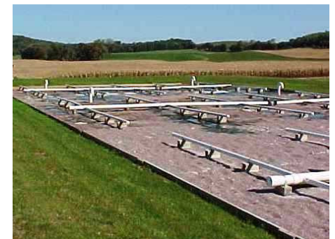
Roxbury Sanitary District #1's Recirculating Sand Filter
