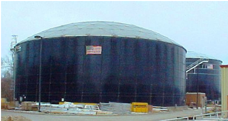
Heart of the Valley's Sludge Storage
